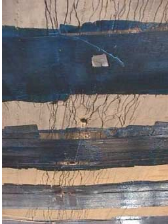
(a) Cracks on deck soffit
