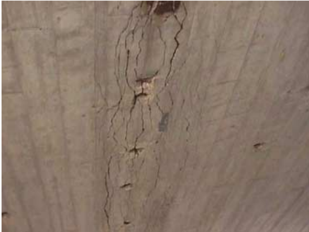
(a) Cracks on the deck soffit testing
