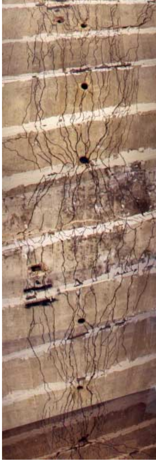
Figure 5.2. Cracks on the soffit of deck 1 after testing to failure.
