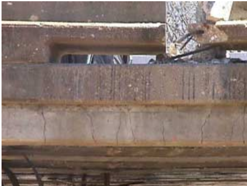
(b) Cracks on the side of the deck
