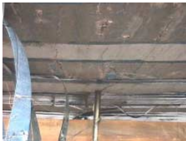
(c) Close up showing peeling of CFRP sheets
