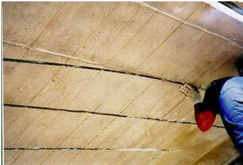
Figure 3.5. Installing the CFRP rods after filling the grooves halfway with epoxy paste.
