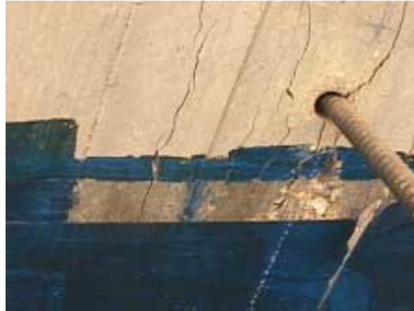
(a) Rupture of CFRP at formlines
