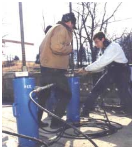
Figure 4.24. Tightening the nuts on the jacks in order to raise the steel girders.
