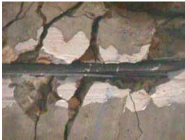
Figure 5.3. Rupture of the mounted CFRP rods at different locations.
