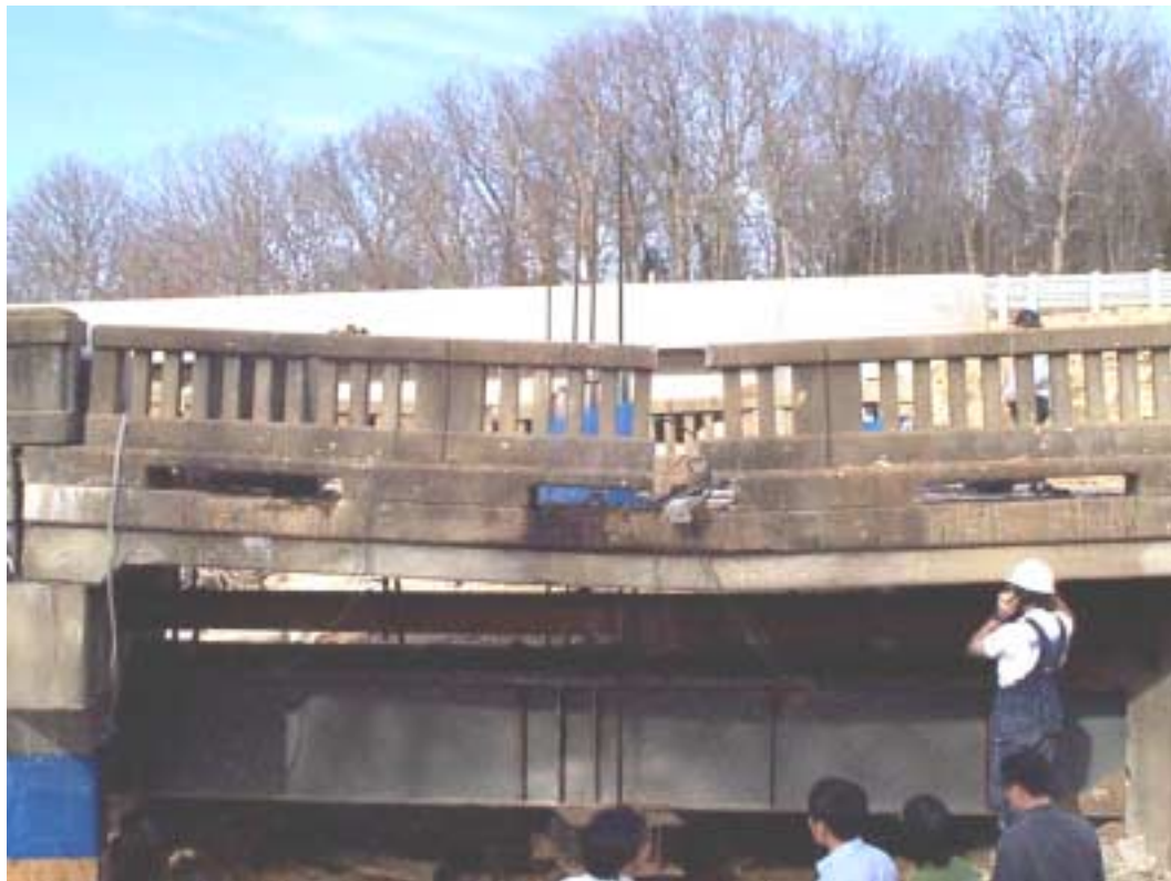
Figure 5.17. Deck 3 at failure.
