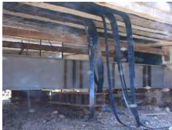
(b) Peeling of CFRP sheets
