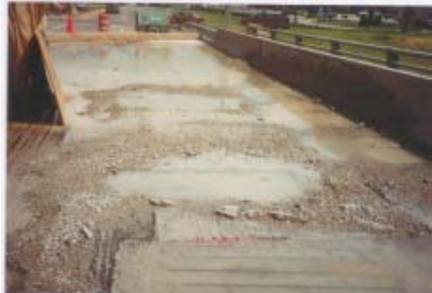
Figure 2: Note the straw bails covered with burlap at the end of the bridge to filter waste water.
