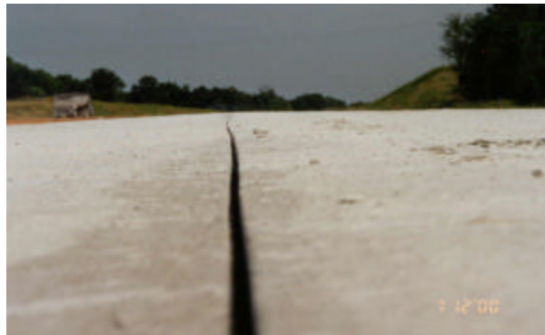
Figure 8. Uneven Longitudinal Sawed Joint Due to Uneven Roadway Edge
