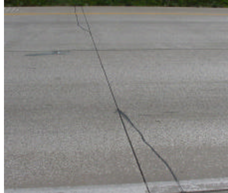
Figure 12. Cracks at Station 74 + 00, RT 44
