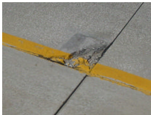
Figure 13. Damage at edge joint intersection at Station 72 + 00, RT 44
