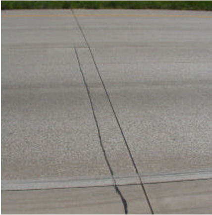
Figure 11. Crack at Mile Marker 94, RT 44
