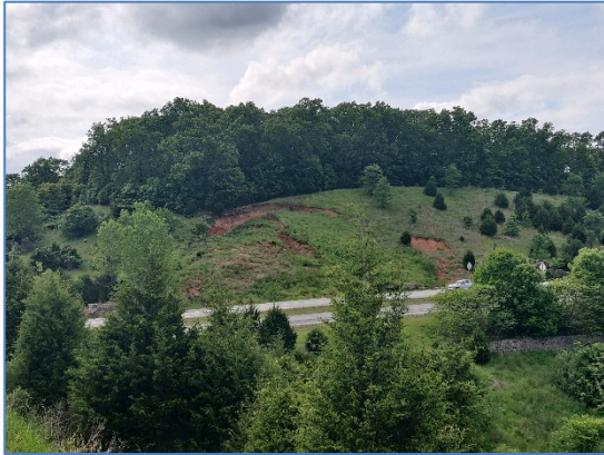
Figure 1: Overview of cut slope landslide and gabion retaining wall system.
