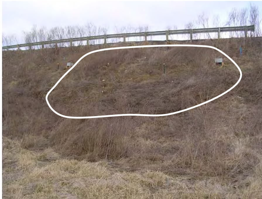
Figure 6.23 Observed failure in slide area S3 at I70-Emma site on January 27, 2005.
