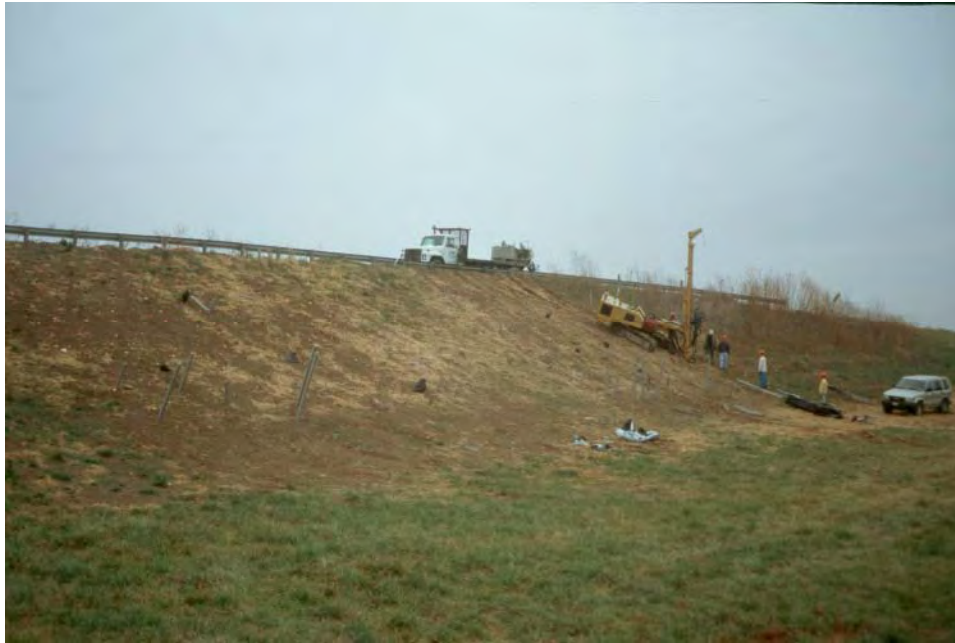
Figure 10.3 Photograph of I70-Emma test set near the end of installation activities for slide areas S1 and S2.
