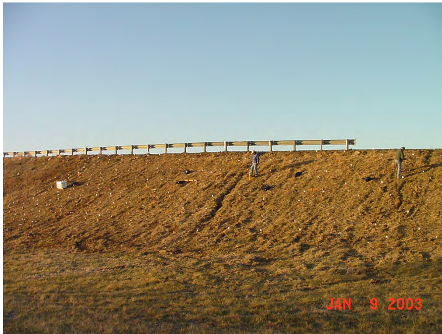
Figure 10.6 Photograph of slide area S3 at the I70-Emma test site following completion of installation activities.
