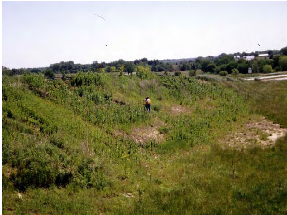
Figure 6.3 Photograph of south side of embankment at I70-Emma site showing slide areas S1 (left), S2 (center), and S3 (right).
