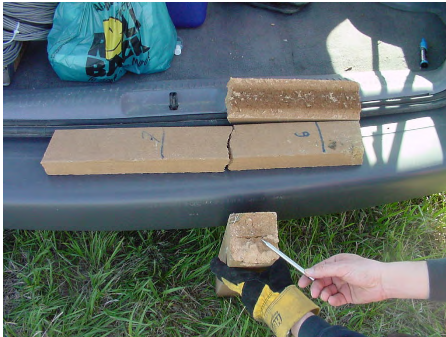
Figure 10.14 Photographs of defective recycled plastic members damaged during installation.
