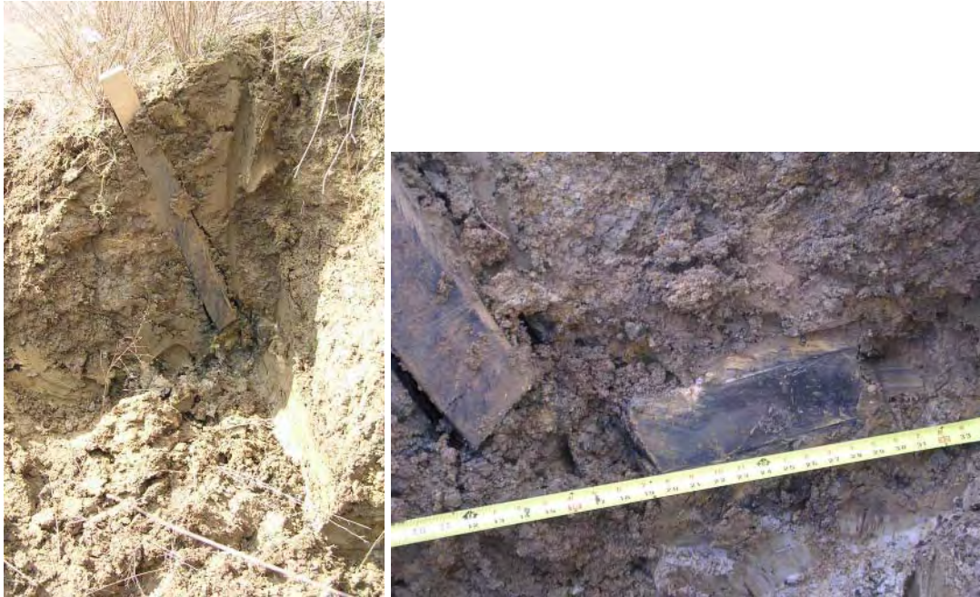
Figure 6.27 Photograph of member M-1 in slope during excavation: (a) entire members and (b) close up of fractured section.
