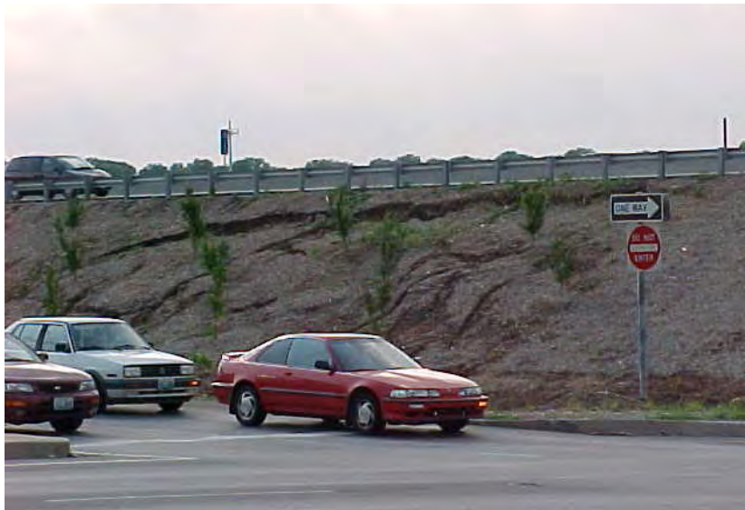
Figure 7.5 Photograph of the I435 Control Slide prior to being regraded for use as a control section.
