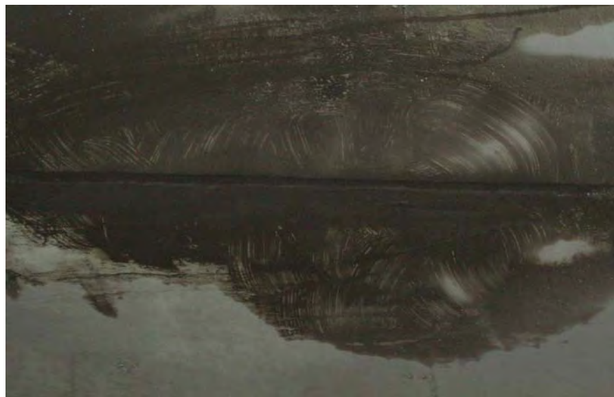
Figure 6 - Close up shows no cracking. Curing compound allowed on this job, but it should be noted that it was done in very mild October weather and was not exposed to sun as it was inside a tunnel.
