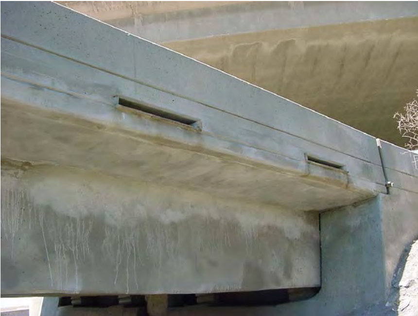
Figure 2 - Bridge A0991 – overhang near NE corner of abutment.
