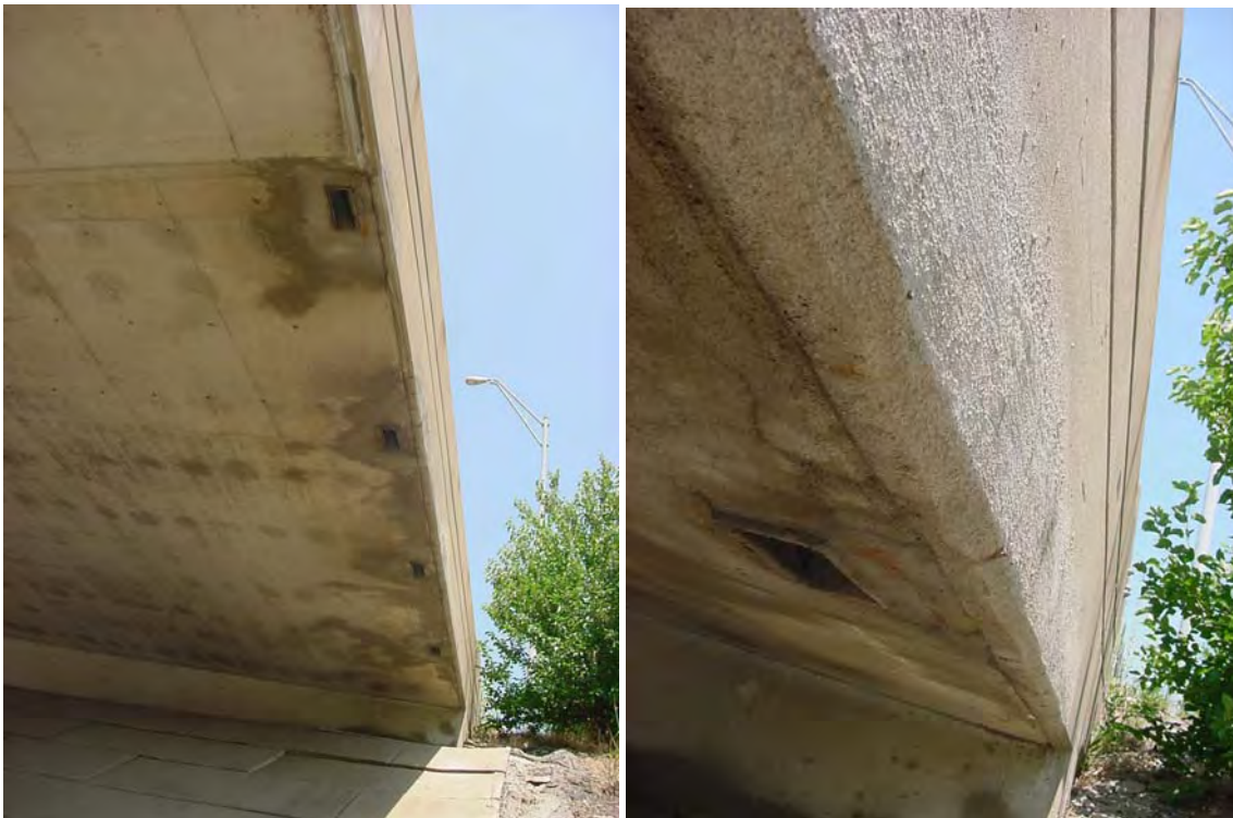
Figure 1 - Br. A2175, shotcrete patches around drains now 8 years old.
