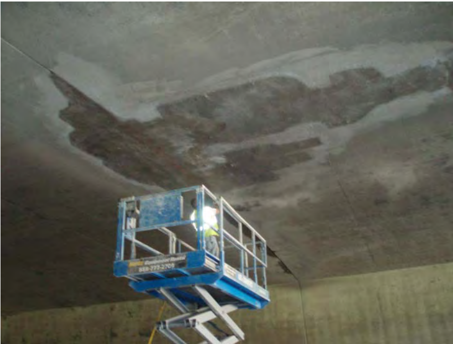
Figure 5 - Repairs on the underside joint of the roof of a tunnel bridge on Project J4I1699, NB I-35 in Kansas City. The dry method using pre-bagged mix did a good job here.
