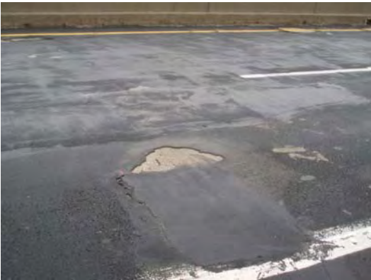
Missing areas of epoxy
