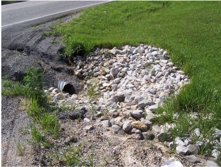
Figure 6.13 Drainage improvements at the intersection of St. Charles Road and Route Z (Rossy et al., 2009).
